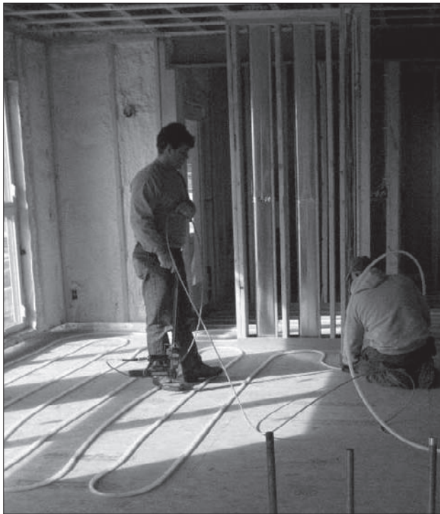
Figure 7. The hydronic PEX tubing was embedded in a 4-inch concrete slab installed over a wood-framed floor.
