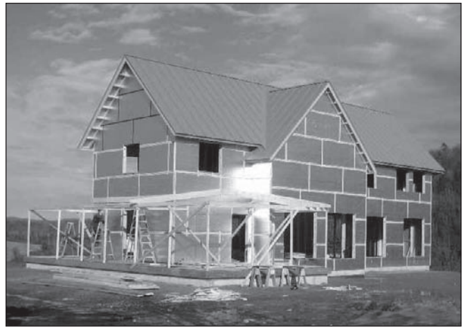
Figure 3. The exterior walls were covered with a layer of 1-inch-thick foil-faced polyisocyanurate foam insulation. Builder Jim Huntington taped the seams with Tyvek tape.
