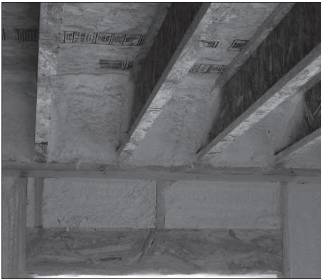
Figure 2. The rim joists at the Pill house are insulated with 5 inches of closed-cell spray polyurethane foam.
