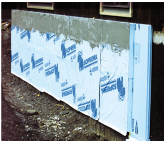
Figure 1. The original EPS foundation insulation was seriously degraded by UV exposure and moisture (top). After cleaning off the stem walls and reapplying asphalt dampproofing, workers installed a double layer of 1½-inch-thick XPS foam, staggering and foaming the joints to minimize air intrusion (above). A peel-and-stick ICF waterproofing membrane protects the new foam from moisture below grade, while a stucco coating protects the above-grade portion from UV damage (right).
